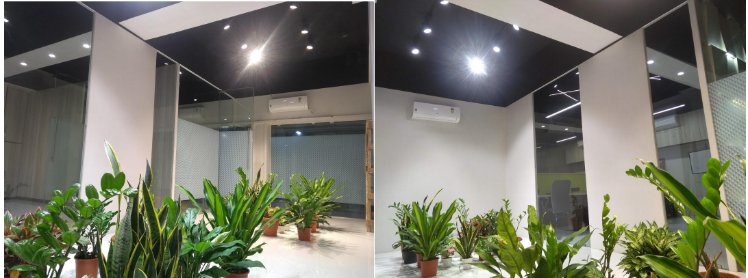
Track lights placed with three luminaires on each side; and a total of six luminaires for each set of plants in 3000K and 4000K respectively
